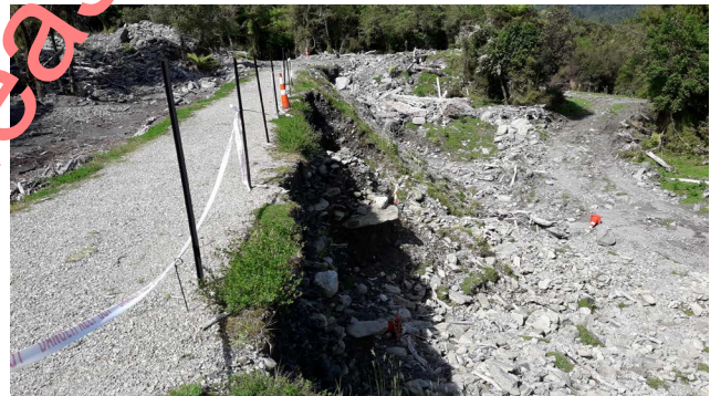
Causeway washout, March 2019
