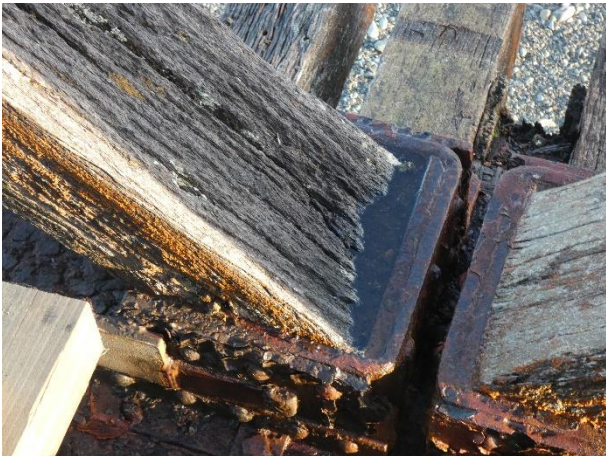
Typical Weathered Timber and Ponding Moisture.
