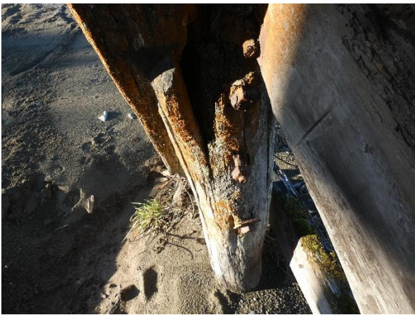
Typical Decay of Pier Piles
