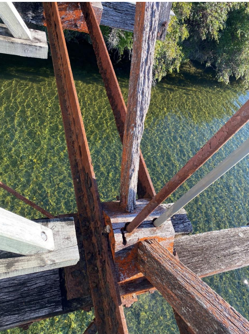
Loss of section on timber strut.
