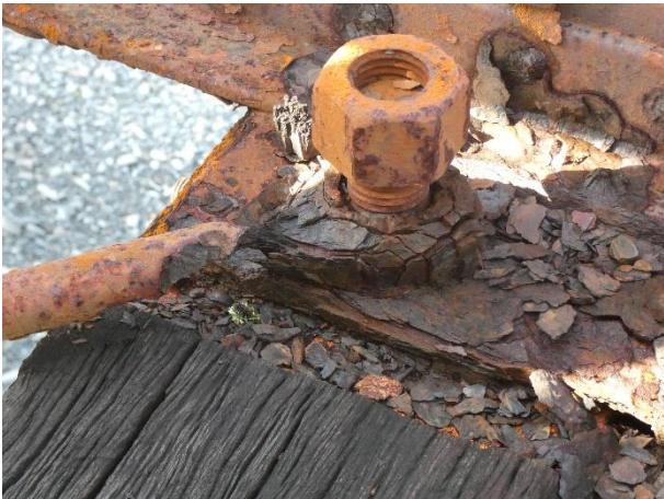
Typical Loose Fixings. Corroded Steel Components.
