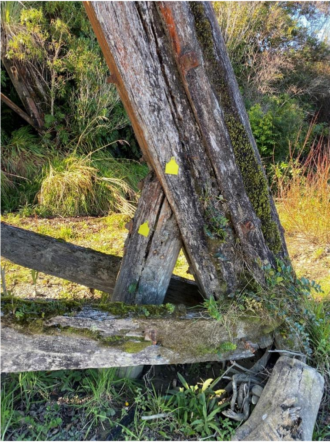
Raking pile timber surface decay
