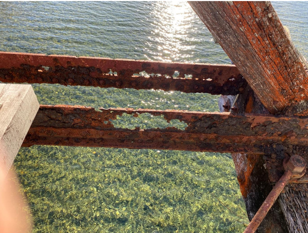
Bottom cord corroded. Needs replacing
