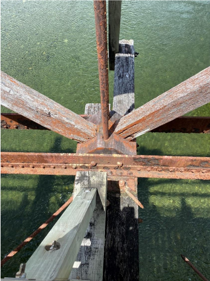
Steel cross bracing corroded. Needs replacing
