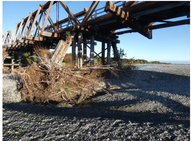
Debris Caught on Piers Causing Local Scour.
