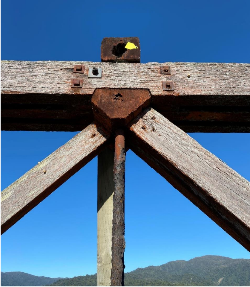
Saddle block with tunnel rot.
