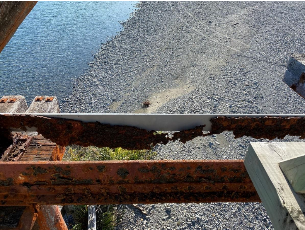
Bottom cord corroded. Previous repair visible.
