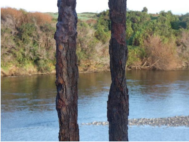
Typical Corroded (Pack Rusting) Hanger Rods – Heavy to Critical Corrosion Shown.
