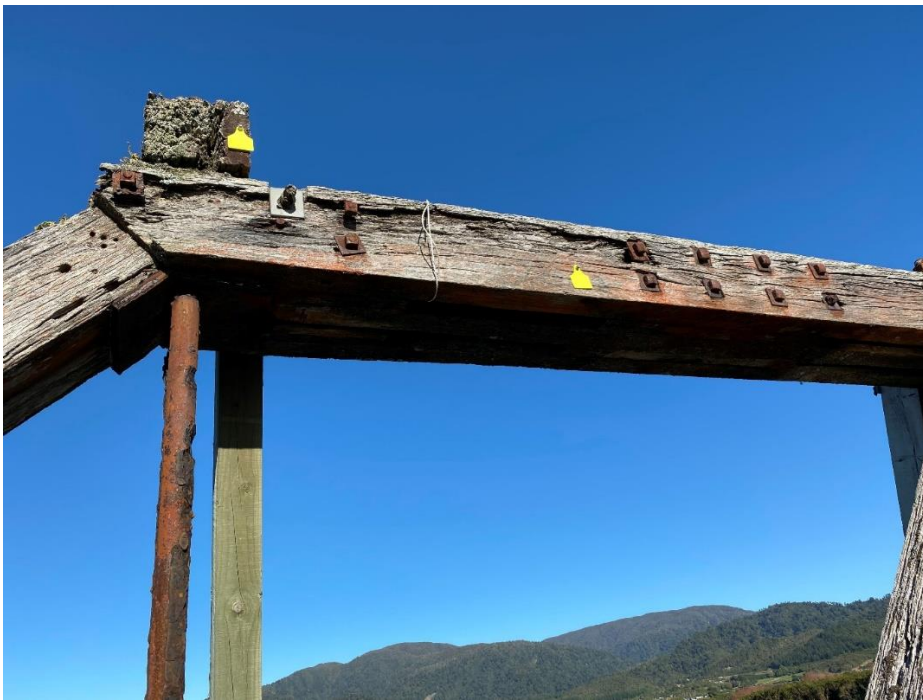
Top Cord Surface loss Saddle block split in timber and timber decay.
