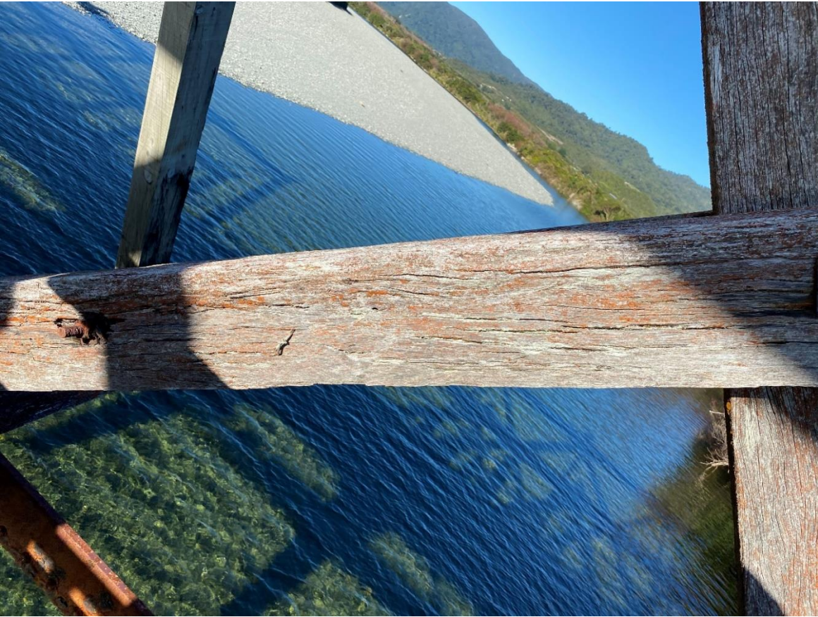
Centre strut timber decay.
