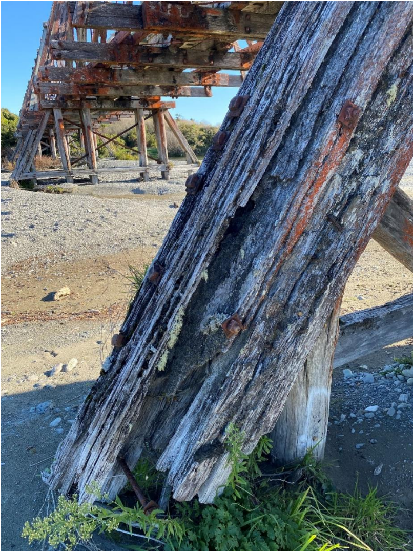
Raking pile timber decay.
