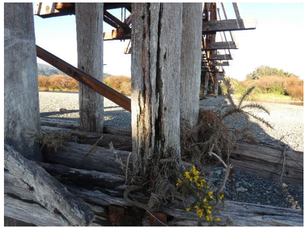
Typical Splitting and Decay of Pier Piles
