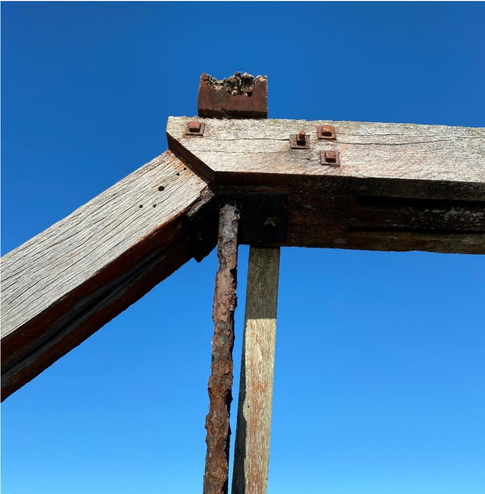
Saddle block timber decay. Tension rod corroded.
