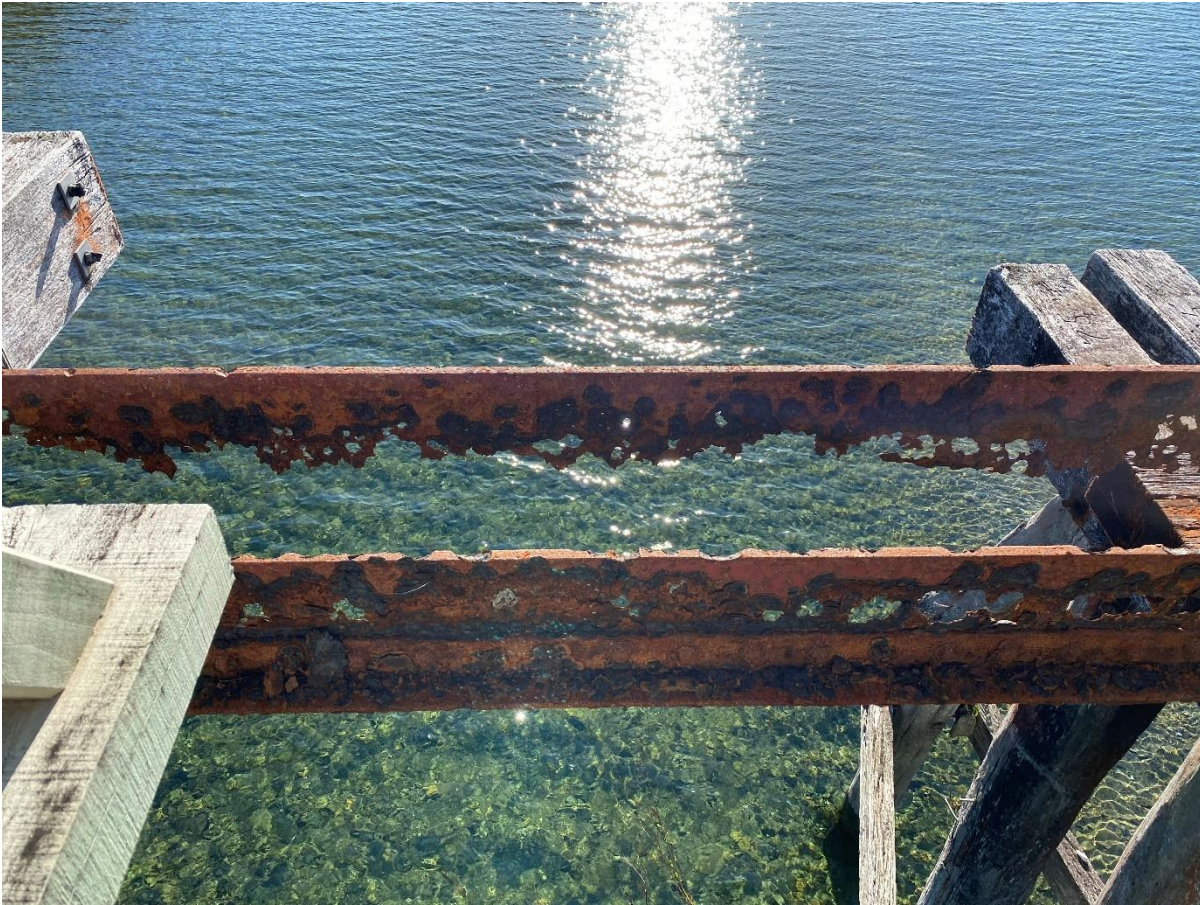
Bottom cord corroded. Needs replacing.
