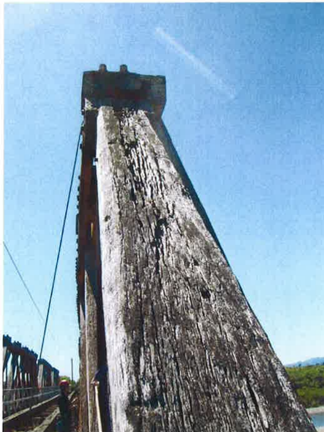
Figure 5-4 : King Strut – Significant Surface Decay, Pocket Decay and Splitting, “Investigate Further”
