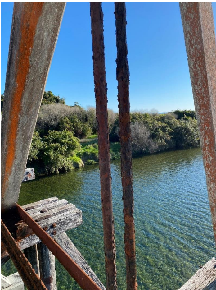
Tension rods corroded. Needs replacing
