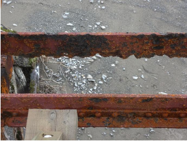
Moderate to Heavy Bottom Chord Corrosion.
