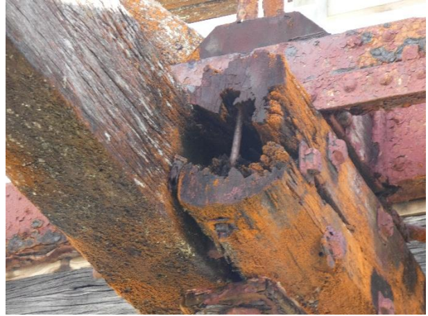
Timber Decay – Heavy to Critical Decay Shown.
