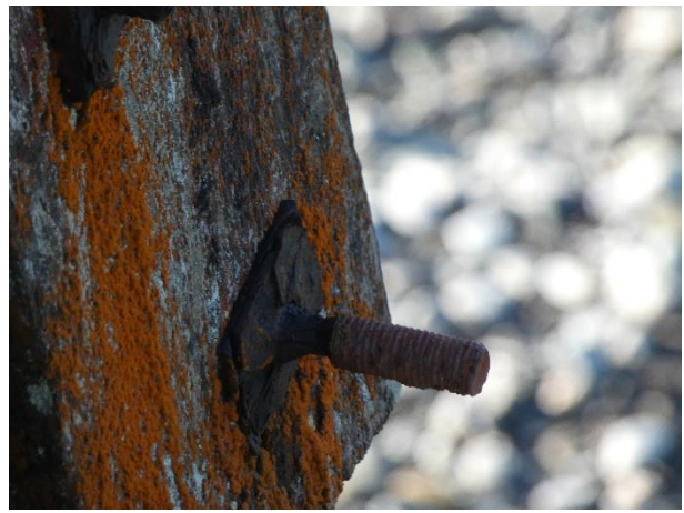
Corrosion and Loss of Fixing Components. Missing Nut and Necked Bolt Shown.
