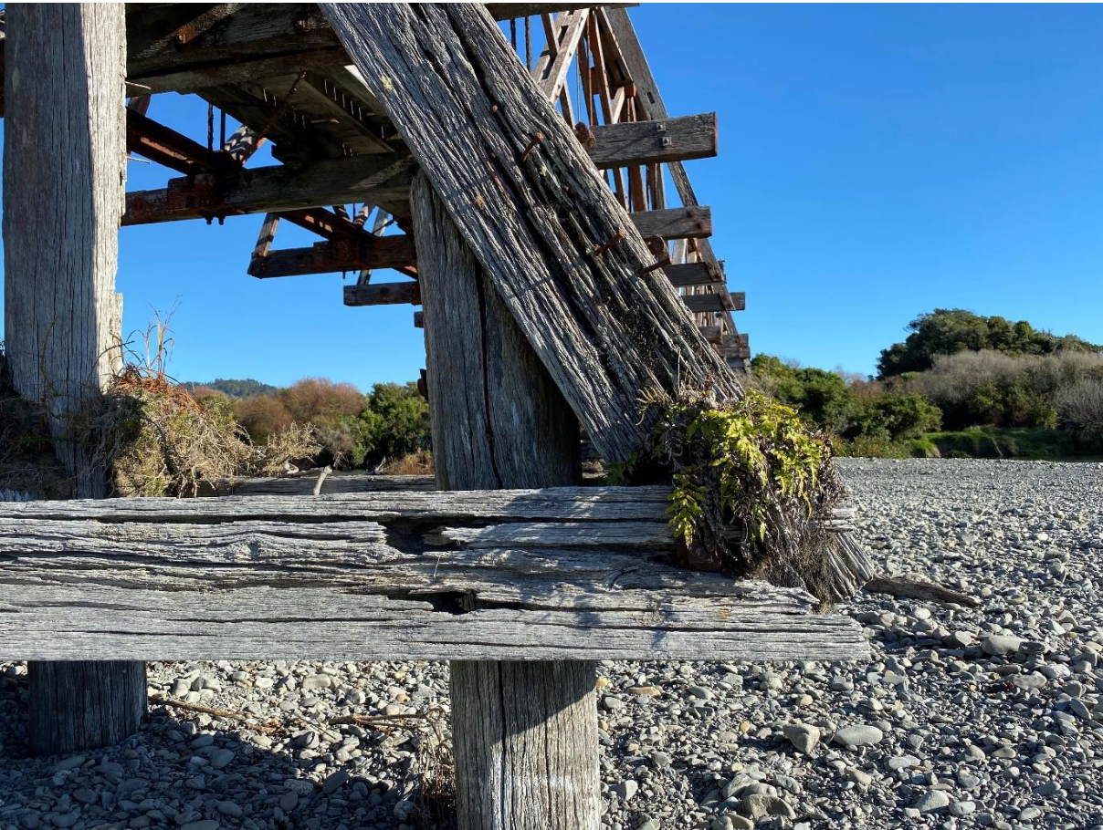
Timber loss and decay.
