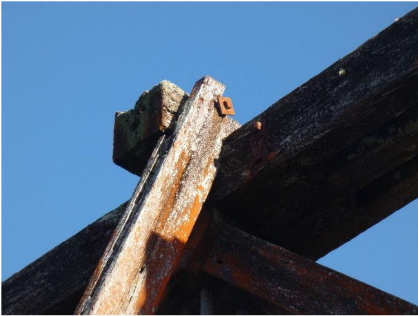
Typical Decay and Loss of Timber Section at Connections – Top of Wind Brace Shown.
