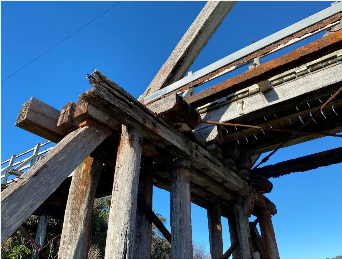
Transom timber end decay Bottom cord corroded. Previous repair visible
