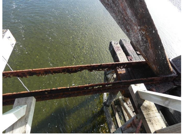
Critical Bottom Chord Corrosion.
