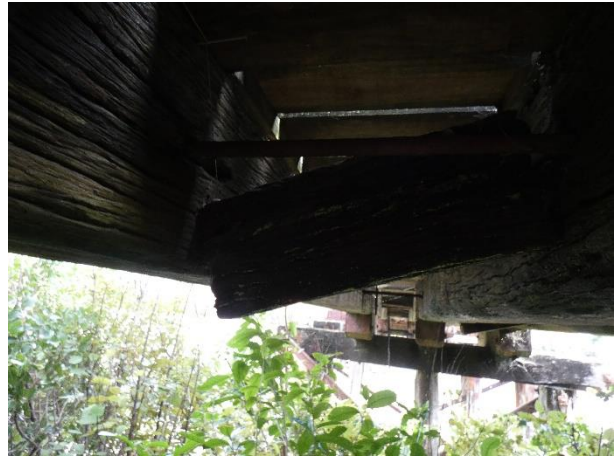
Dislodged and Missing Timber Bracing Blocks Typical.
