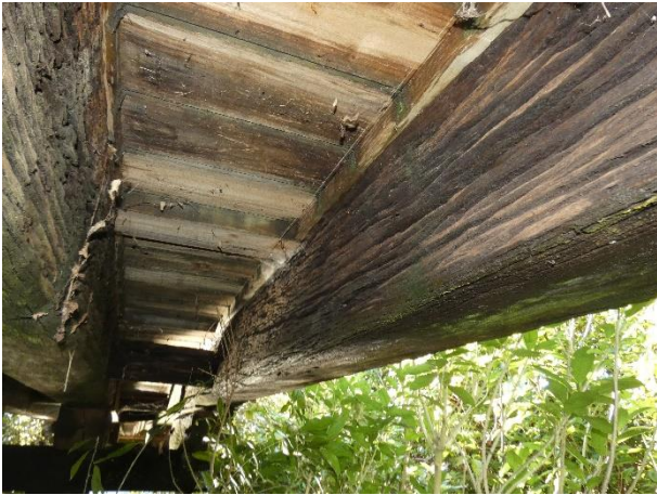
Moisture in Timber Components. Reduced Air Flow for Drying due to Vegetation.
