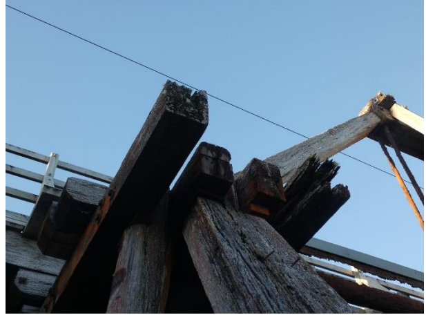
Typical Decay of Pier Cap Timbers
