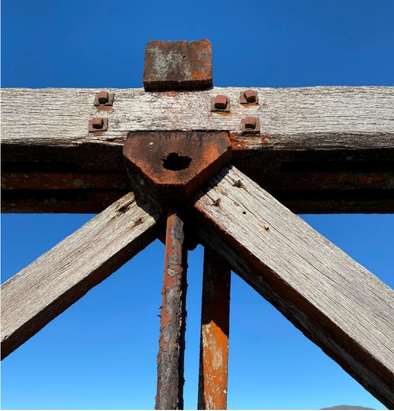
Tiber A block with tunnel rot.
