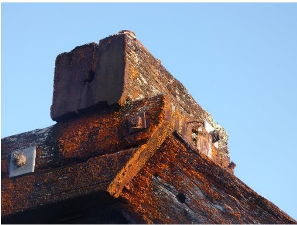
Typical Timber Splitting – Top Chord Shown.
