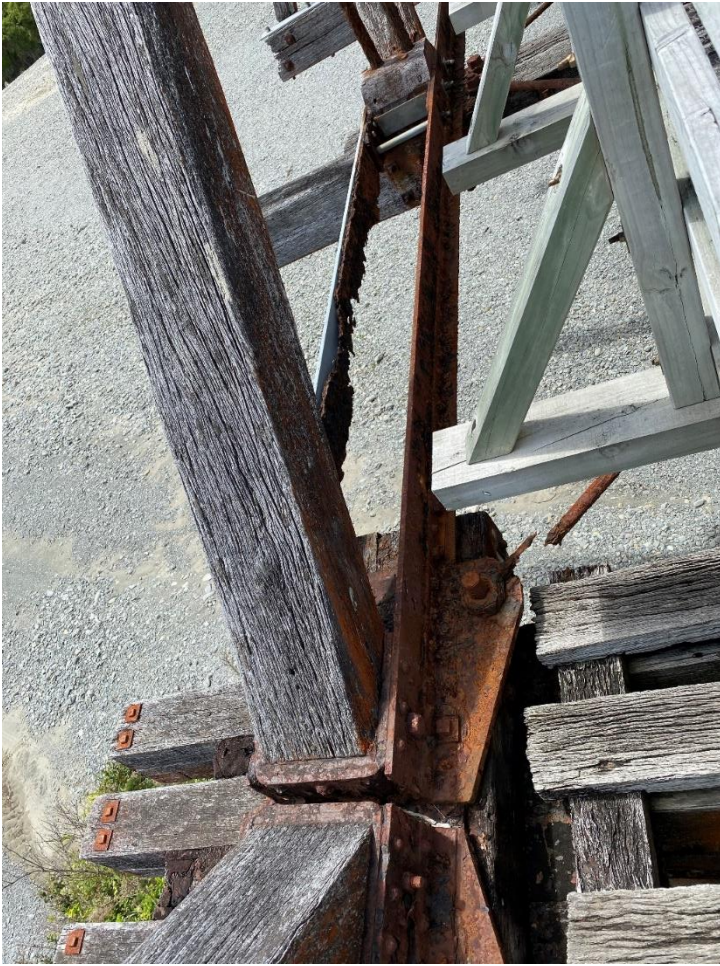
Bottom cord corroded, needs replacing. Cross bracing corroded needs replacing
