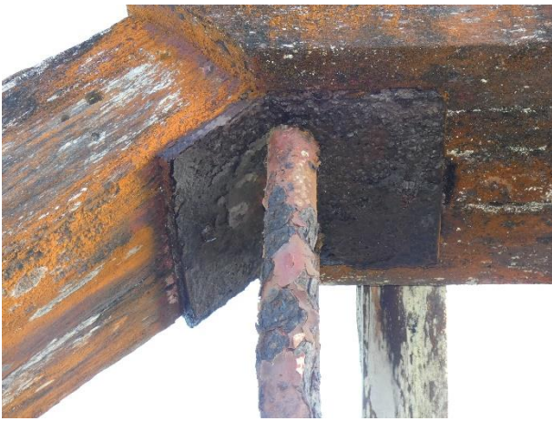
Corrosion of Truss Connection Plates.
