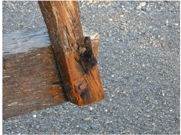
Typical Decay and Loss of Timber Section at Connections – Bottom of Wind Brace Shown.
