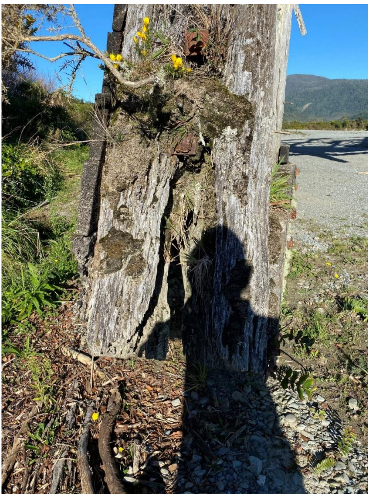
Raking pile timber split and timber decay.
