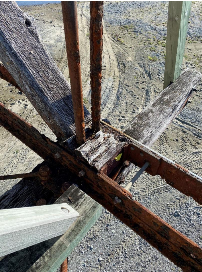
Timber thrust block with timber decay.
