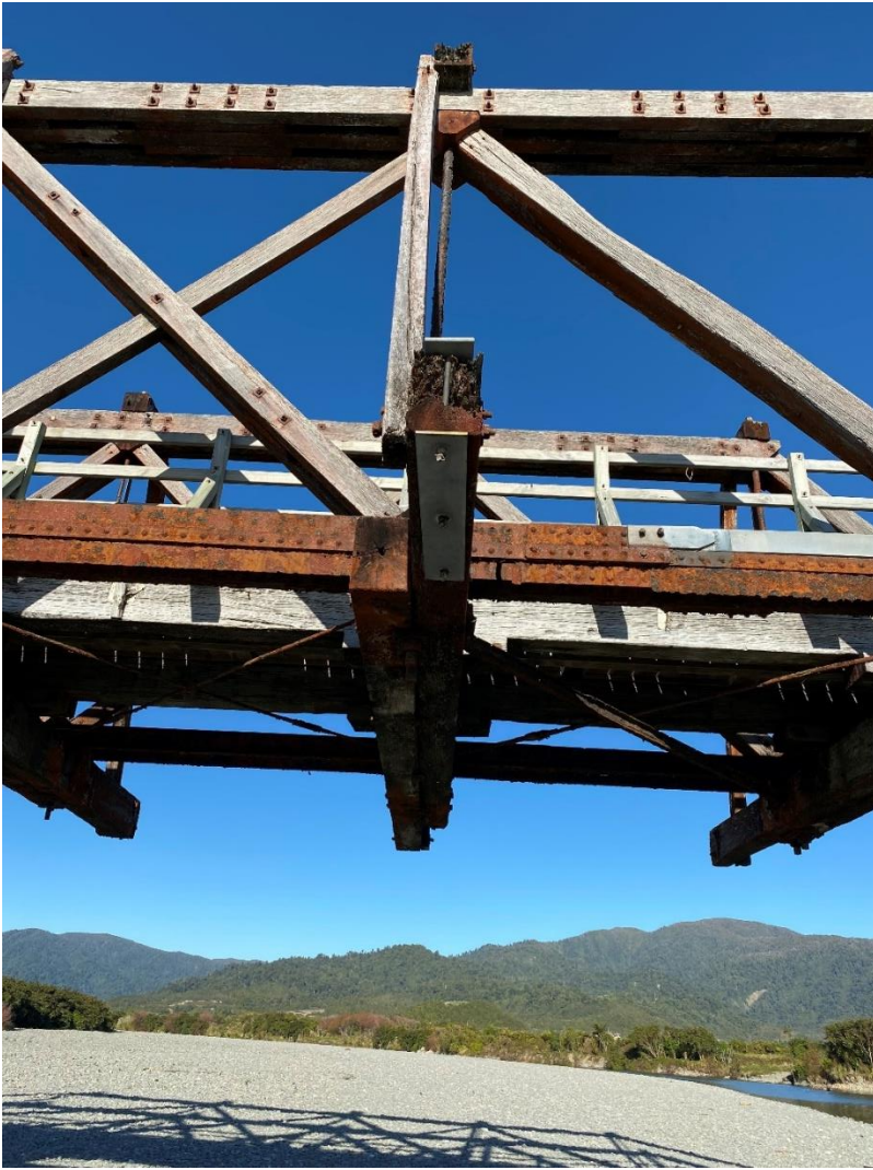
Previous repair to transom end. More timber decay present
