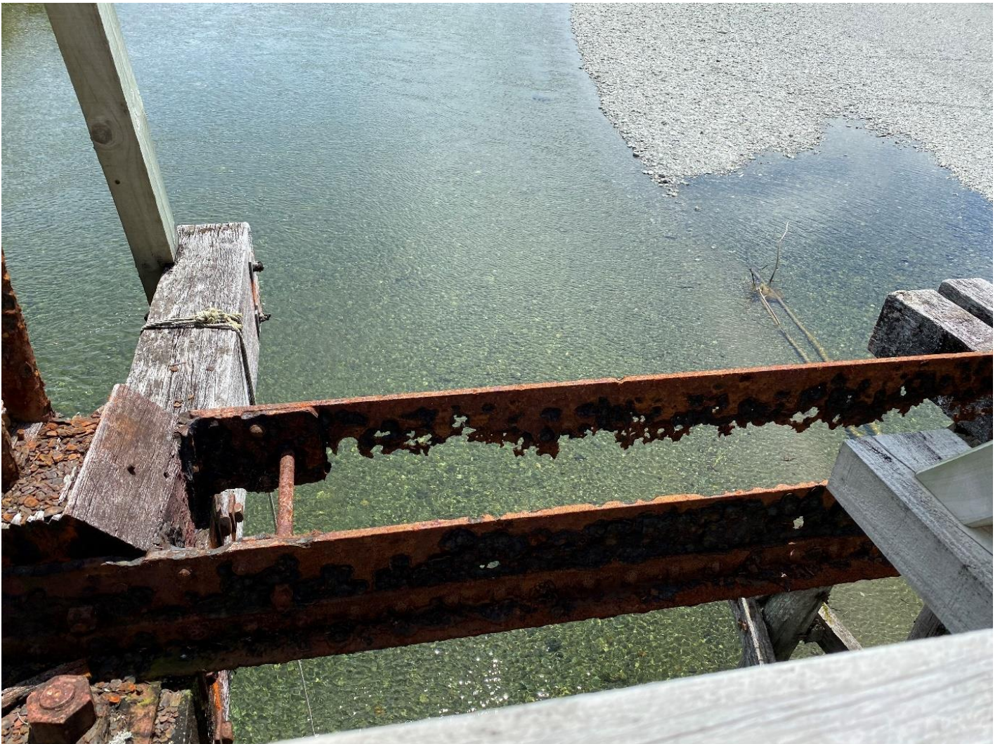
Bottom cord corroded, needs replacing
