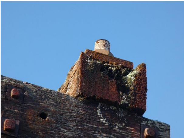
Typical Decay of Top Blocks.
