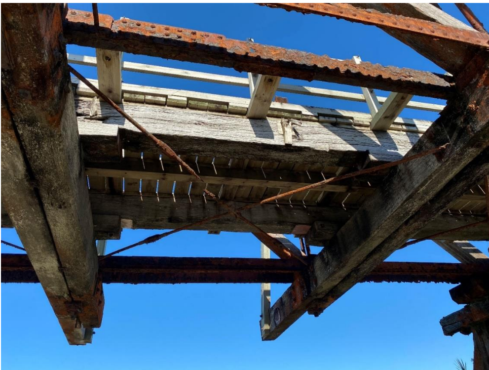
Steel cross bracing needs replacing
