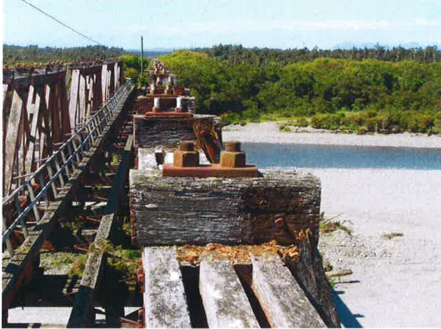
Figure 5-3 : Lateral Braces – Members Completely Decayed at Ends, “Requires Replacement”
