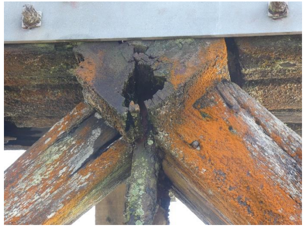
Typical Heavy to Critical Decay of 'A' Block.
