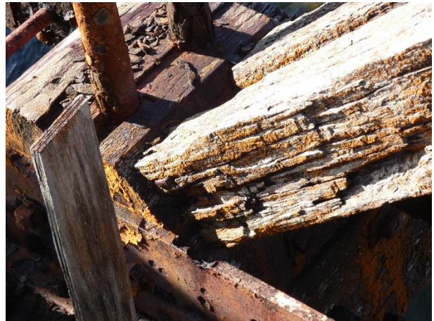
Typical Weathered Timber.
