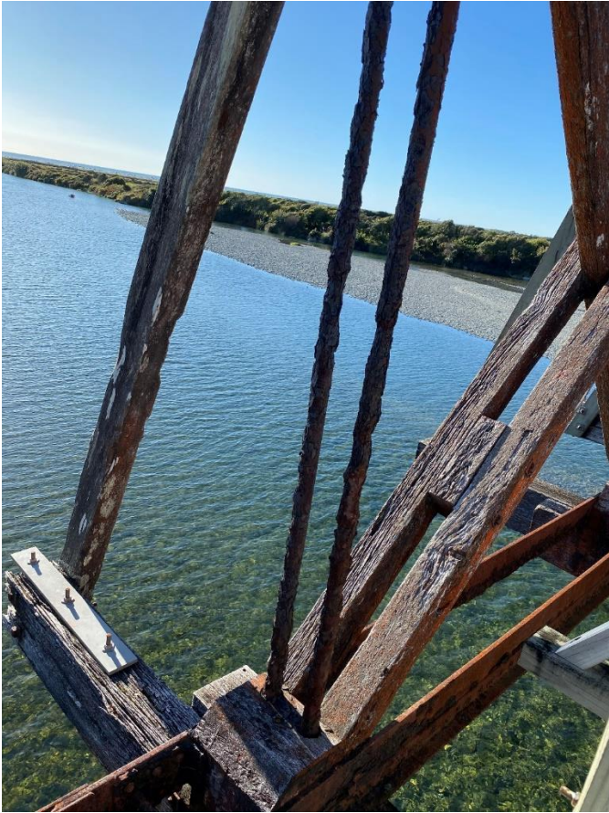
Tension rods corroded. Previous repair to transom. Needs more repairs. Decay to timber strut.
