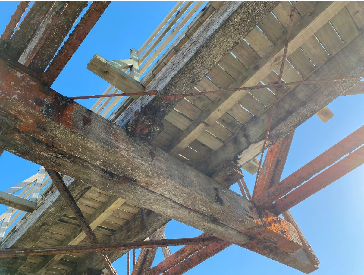
Cross bracing corroded away.
