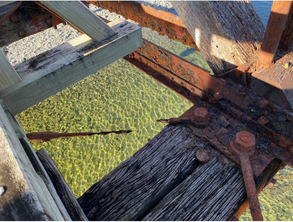
Steel cross bracing corroded. Needs replacing
