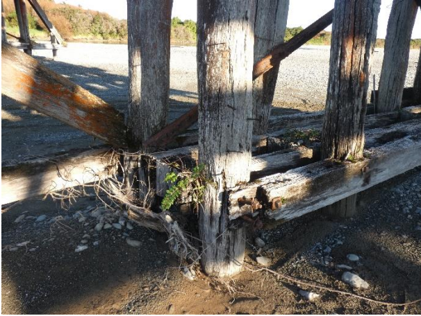
Missing Pier Waling Timbers
