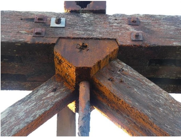
Typical Moderate Decay of 'A' Block.
