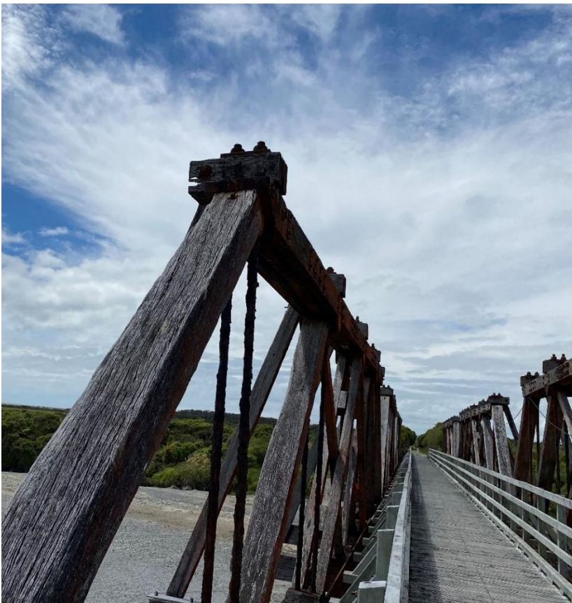
Saddle block decay and split.
