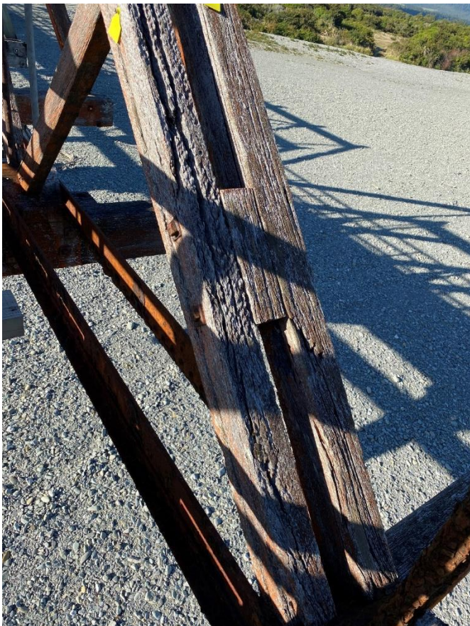
Surface loss on timber strut
