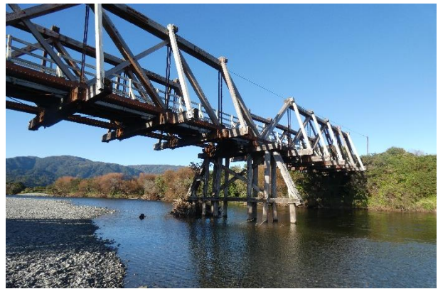
Pier G and Underside of Span G-H not inspected due to Channel Location. Main Channel is Deep. Pile Embedment Depth Unknown.
