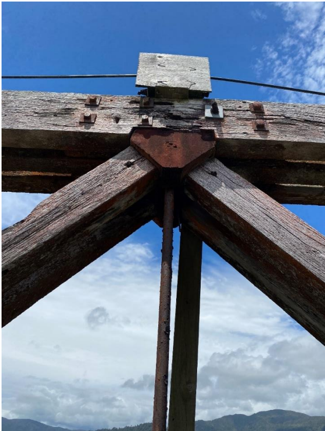
Saddle block needs replacing.
