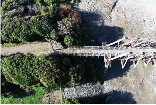
Approach Spans Shrouded in Dense Vegetation. Northern Approach.
