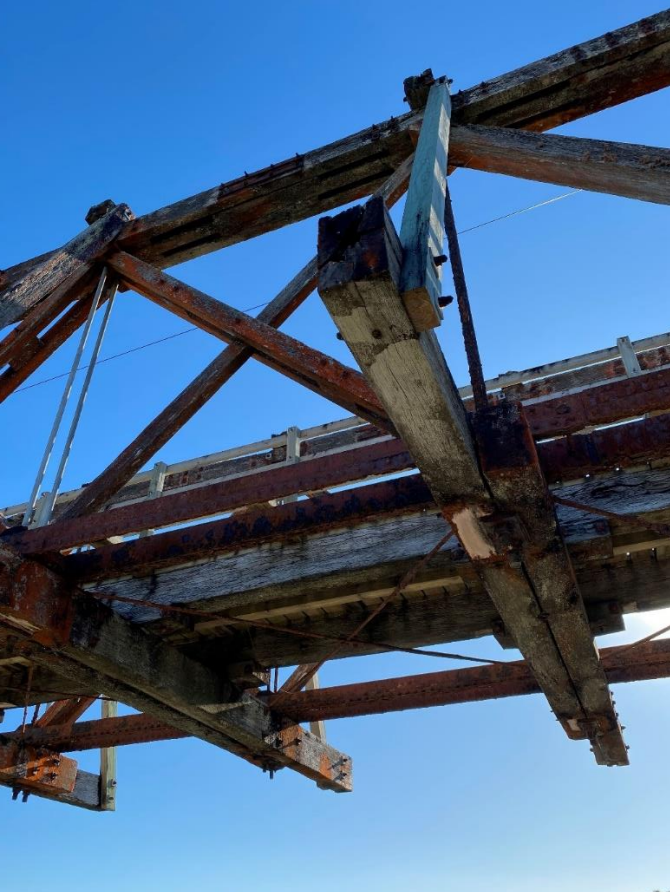
Transom end timber decay.
