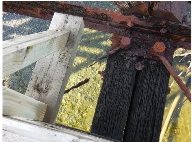
Widespread Loss of Deck Bracing Due to Corrosion.
