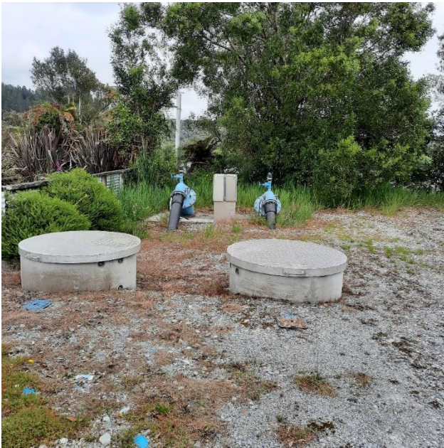
Figure 3-5: River Intake Pumps.
