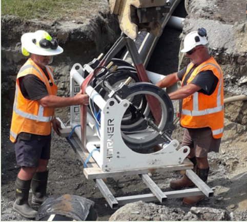
Coast to Coast Team carrying out PE pipe welding at a job in Christchurch.
